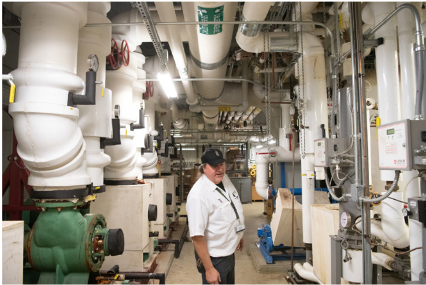
JOE PFEIFFER CHECKS THE CHILLER RETURNS UNDERNEATH THE PHARMACY SOUTH BUILDING.
