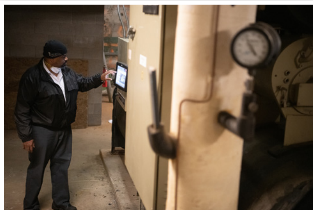
HAMLIN CHECKS SYSTEMS DURING HIS PORTION OF NIGHTLY ROUNDS IN THE BASEMENT OF THE SCHOOL OF NURSING BUILDING.
