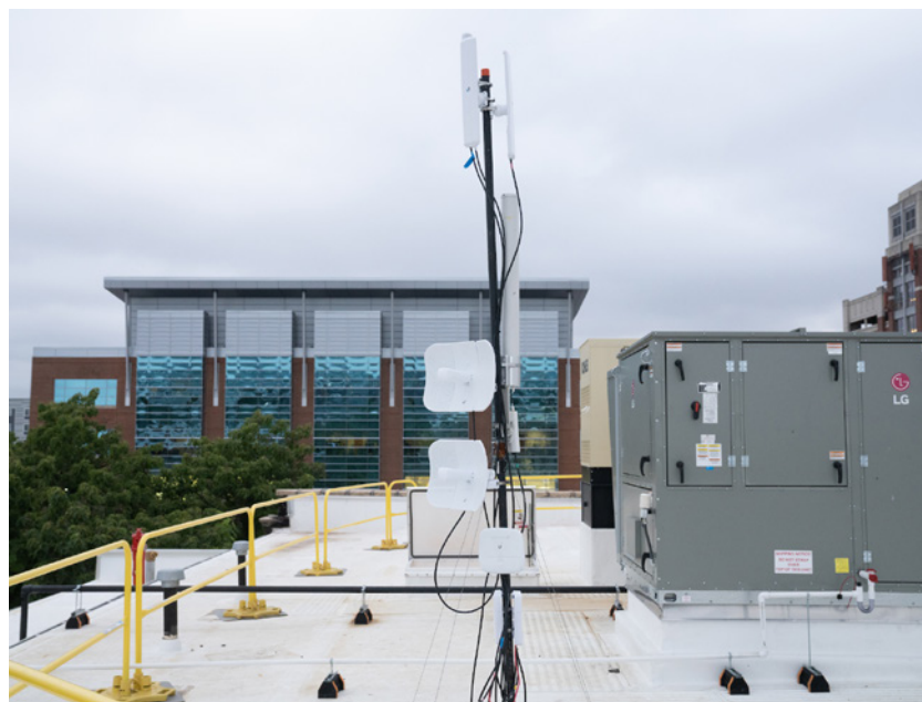
SECTOR ANTENNAS WERE INSTALLED ATOP THE NEW COMMUNITY ENGAGEMENT CENTER BUILDING AS PART OF UMB'S PARTNERSHIP WITH PROJECT WAVES TO PROVIDE WEST BALTIMORE RESIDENTS WITH FREE INTERNET ACCESS.
