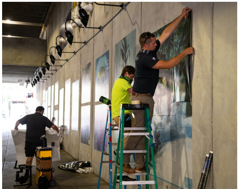
WORKERS INSTALL THE '1807' PIECES, WHICH WERE PLACED ON VINYL APPLIQUES AND ARE ILLUMINATED BY LED SPOTLIGHTS.
